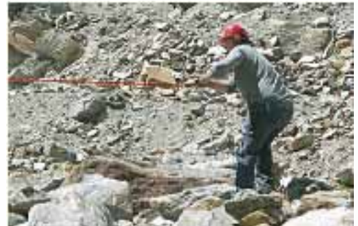
12 The cracking is triggered from a safe distance by means of the pull rope: wearing of hard hat, ear plugs, protective glasses and safety shoes is obligatory.
